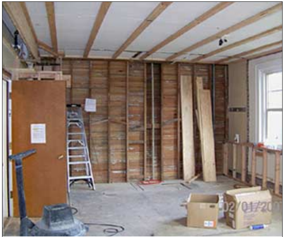
The Odd Fellows Home Beauty Salon should be open in the very near future. If you would like to make a contribution to the remodeling of the Beauty Salon, see story at left.
