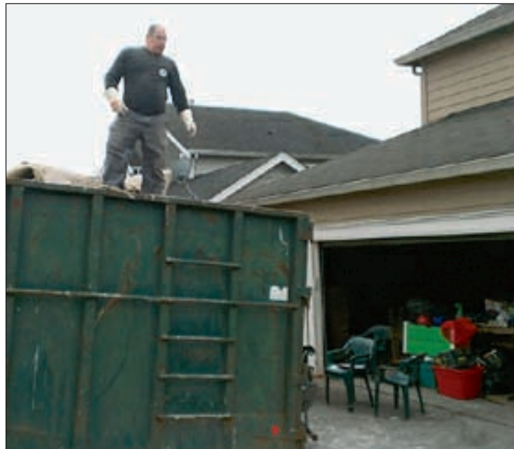
Buckley IOOF Lodge #75's Vice Grand Doug Smith helps fill a huge dumpster with debris following a major fire at Brother Ari Rogaway's home. Several Buckley member helped clean up the mess.
