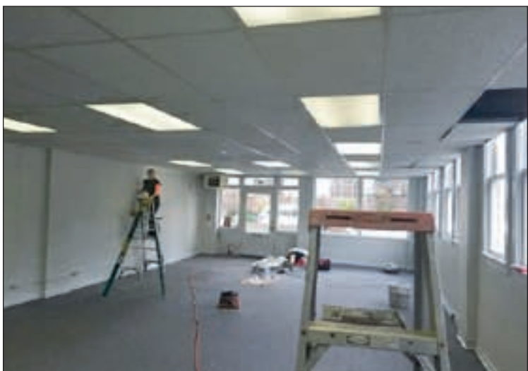
Joanne Balmert works on painting the "vault room." It looks pretty big, doesn't it?
