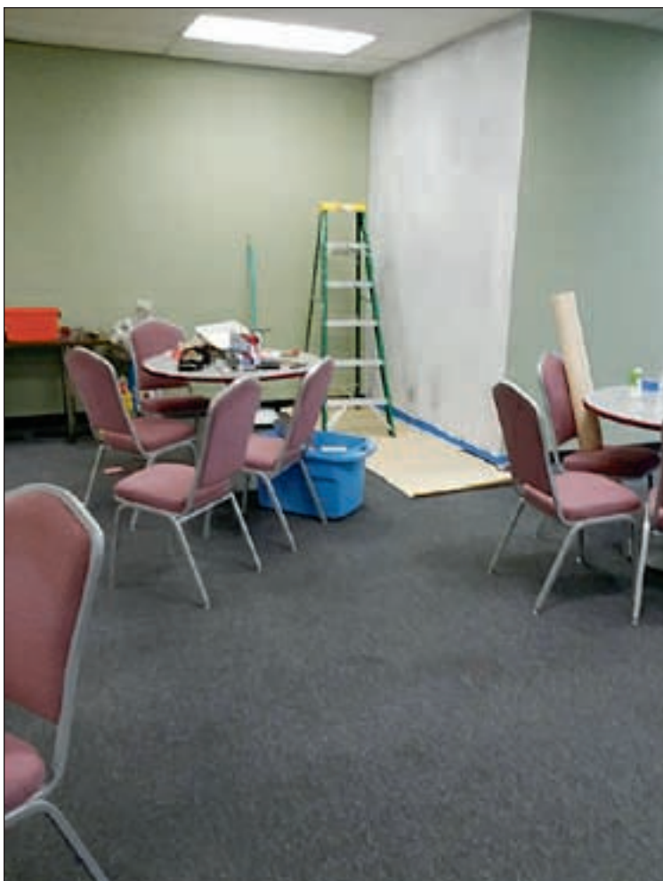
A nice coat of white paint replaced the pink which looks so much brighter.
